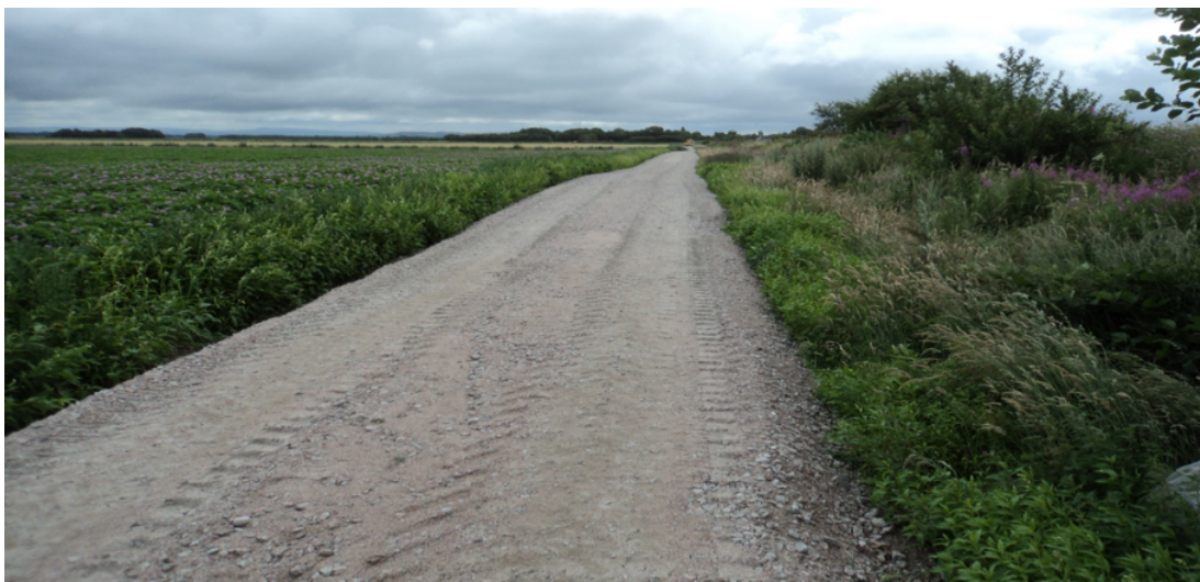
Figure 5: Top – Reduced depth of cover from vehicular movement identified Middle – Cellular confinement system installed to prevent further erosion Bottom – Depth of cover reinstated with material appropriate for land use
