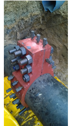
Epoxy filled tee (by Team Inc)
