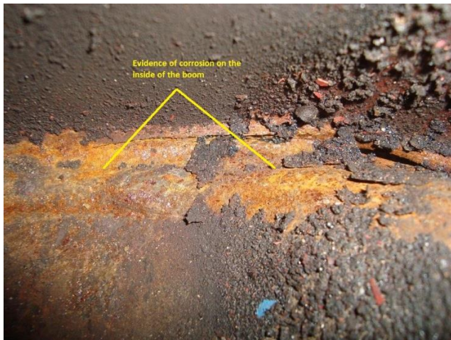
Showing close-up of corrosion
