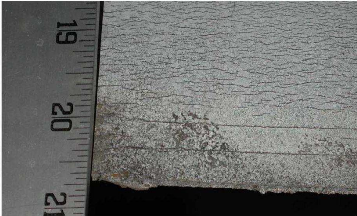
Figure 1 SCC colonies (Both high pH and near neutral pH SCC appear similar from a visual assessment)
