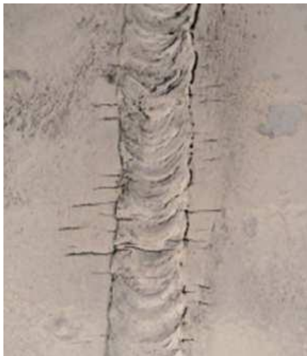
Figure 5 Near neutral pH SCC in vicinity of girth weld
