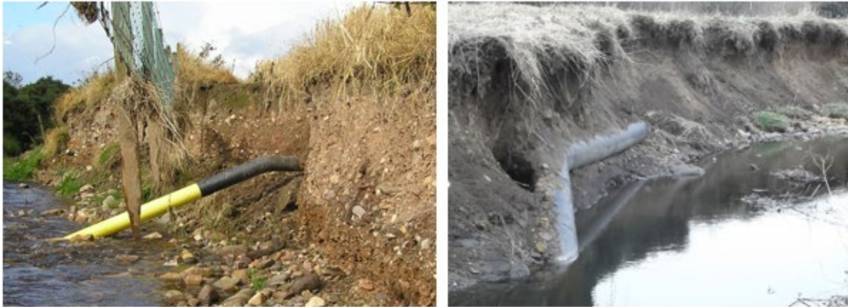
Figure A-7: Free Spanning Pipelines Due to Horizontal Channel Scour
