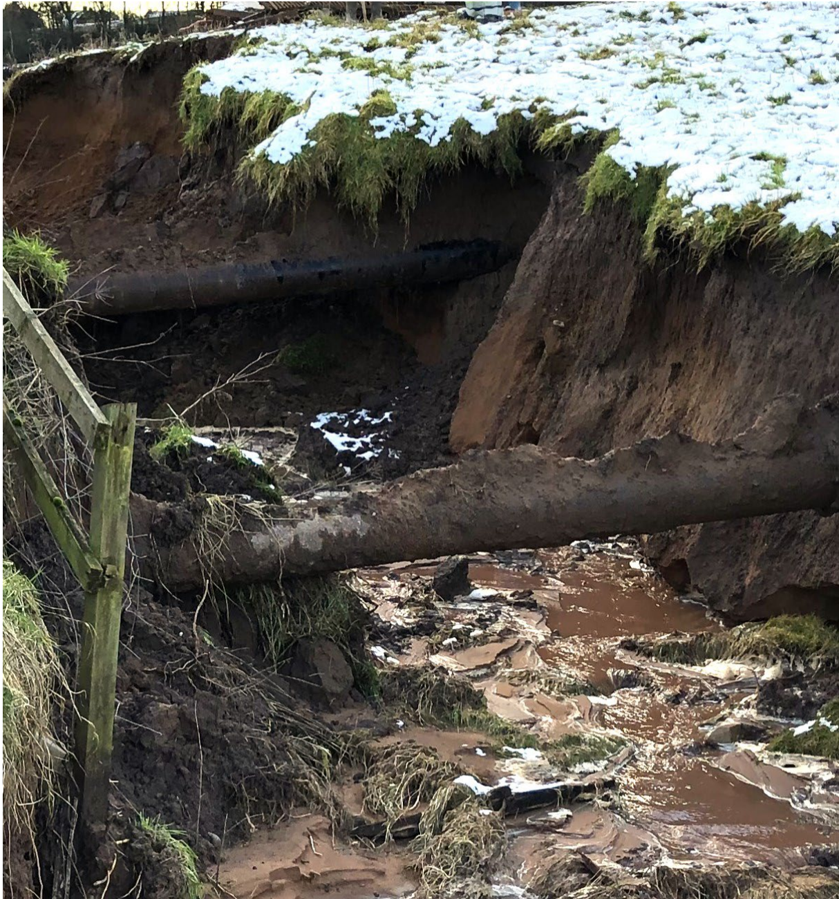
Figure A-5: Washout of Soil During Flooding
