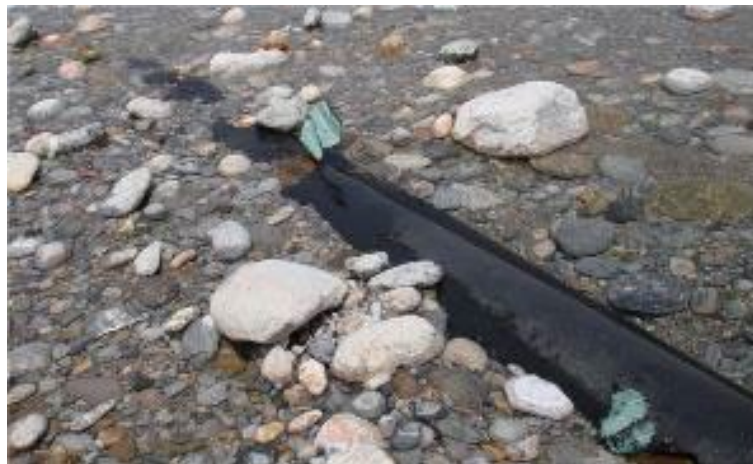
Figure A-8: Pipeline exposure due to vertical channel erosion
