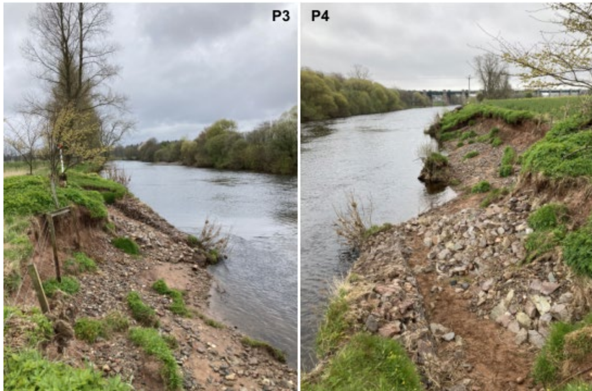
Figure A-2: Left from P3 - View of Erosion on Right (South) Bank Looking North-West (Upstream) Right From P4 - View of Erosion on Right (South) Bank Looking South-East (Downstream)
