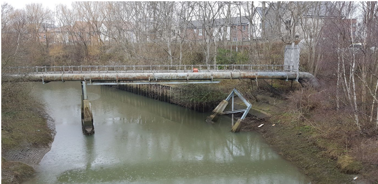
Figure A-12: Loss of Pipeline Support at Overcrossing
